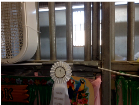
Duct Tape for electric cord from Box Fan
